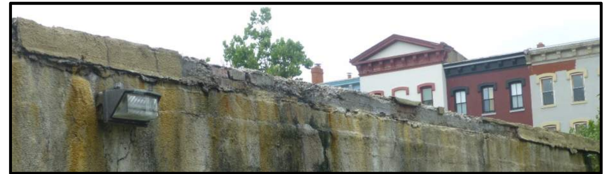
Figure 29 - Roof Level Parge Spalls
