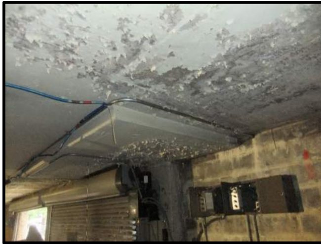
Figure 5 – Peeling Paint (Entry Level)
