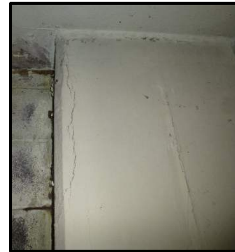
Figure 17 - Column Crack (Entry Level)
