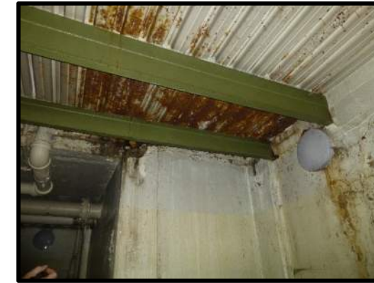
Figure 22 - Corroded Metal Deck (Northwest Stair)
