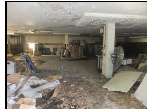
Figure 1 – Entrance Level Stored Items
