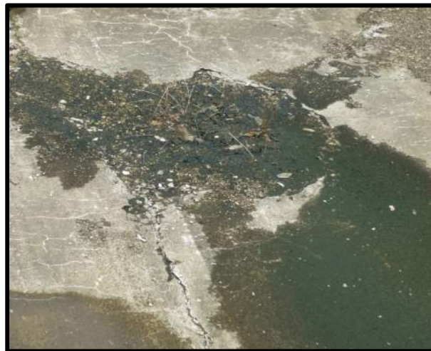
Figure 33 - Lower Roof Ponding and Typical Clogged Drain
