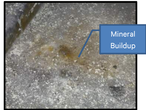
Figure 21 – Mineral Buildup (First Floor Ramp)
