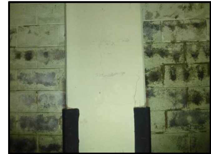
Figure 18 - Column Crack (Entry Level)
