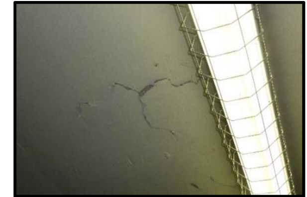
Figure 8 – Typical Ceiling Spall
