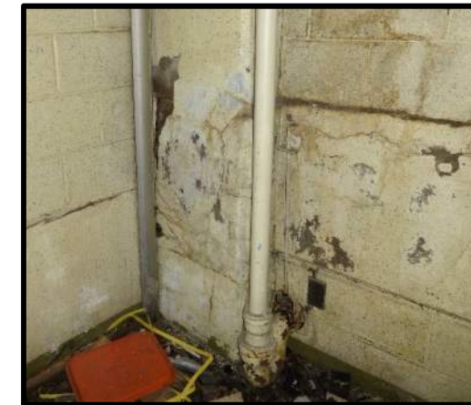
Figure 24 - Ground Level Damage (Southwest Tower)
