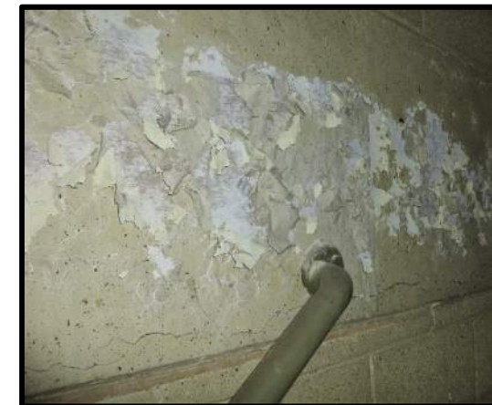
Figure 25 – Typical Upper Level Damage
