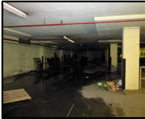
Figure 11 - Ponding (Entry Level)
