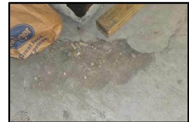
Figure 10 – Typical Floor Spall
