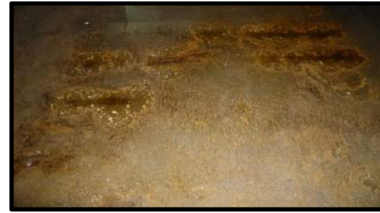
Figure 12 - Exposed Rebar (Entry Level)
