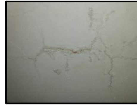
Figure 15 - Typical Ceiling Cracks
