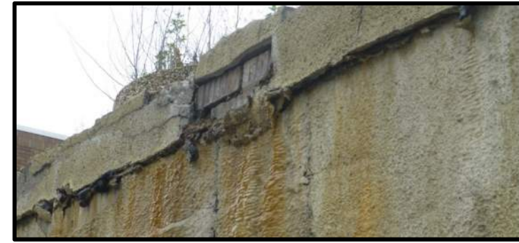
Figure 28 - Efflorescence and Failing Sealant
