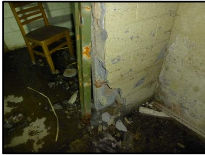
Figure 26 - Damaged CMU Wall (Southwest Tower)
