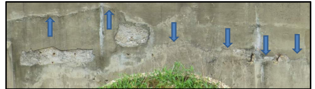
Figure 35 - Typical Roof Wall Spalling and Exposed Rebar
