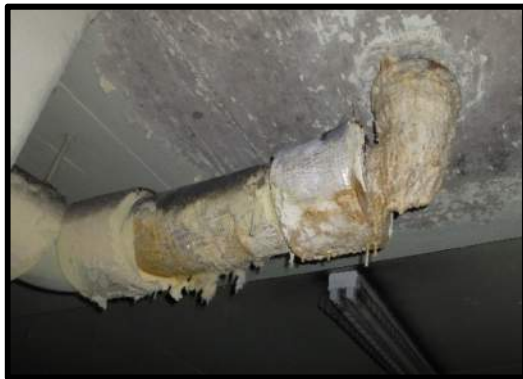
Figure 20 – Efflorescence on Roof Drain
