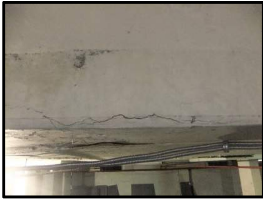
Figure 19 – Beam Cracking with Slab Spall Beyond (Entry Level)
