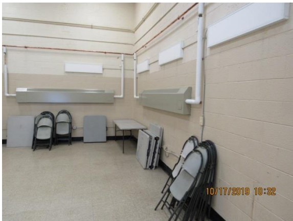
New heating convectors and insulated piping at Stoddert Terrace Community Center
